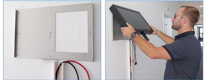
Connections separated from the monitor
